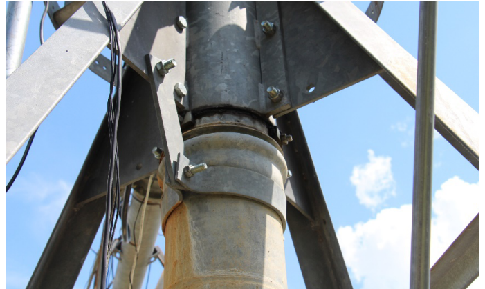
Figure 19. Visible signs of wear and use are often evident on the pivot point. In some cases, a closer inspection is needed. Carefully consider whether repair or replacement is needed.
