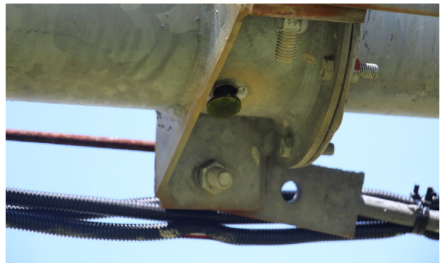
Figure 11. The drain valve for one of the pivot towers. In this case, the valve is open because there is no water in the system.
