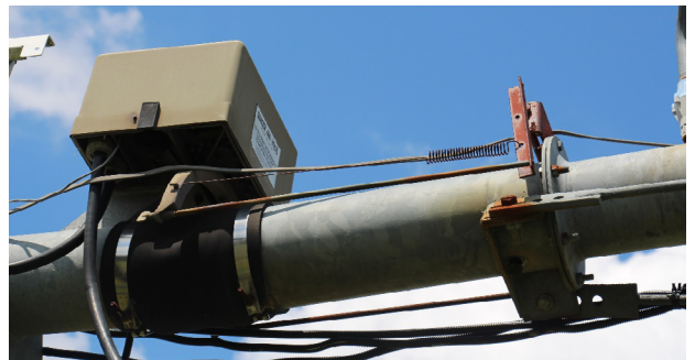
Figure 12. An alignment switch located at the connection point between two pivot towers. Ensure that all components on the alignment system are in working order. Replace any components that appear worn and may not last through the season.
