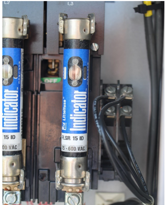
Figure 4. Notice the visual indicator on these main power fuses in the control panel. If a fuse is questionable, power the system down, remove the fuse, and check connectivity with an ohm meter. If it does not have a visual indicator, testing resistance/connectivity is another way to check whether a fuse is operational.
