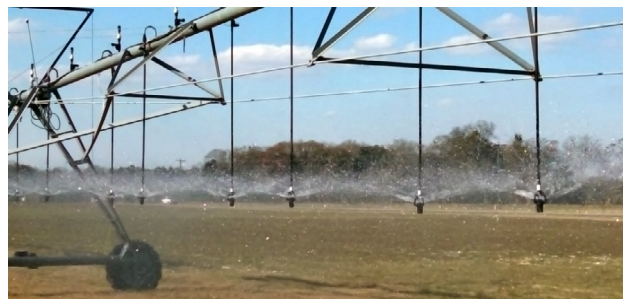
Figure 9. Nozzles operating on a center pivot system. In some instances, uniformity or other nozzle-related issues can be observed through visual assessment. Sprinkler uniformity can be quantified using the methods described in UGA Extension Circular 911.
