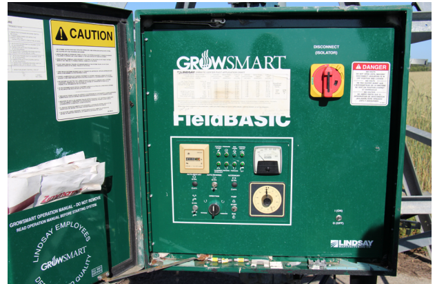
Figure 1. The main control panel on the irrigation system. Ensure power is disconnected and all switches are turned to the “off” position before opening.
