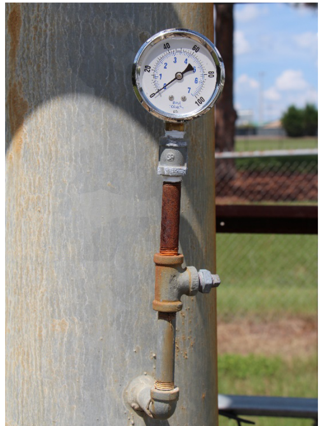
Figure 5. The main pressure gauge at the pivot point. The pressure should be the highest at this location and is an important position to verify proper pressure for pivot performance.
