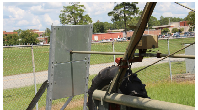
Figure 13. The stop and safety switch on a pivot. In this case, if either switch malfunctioned, the pivot would walk over the fence and into the road—a very dangerous situation.
